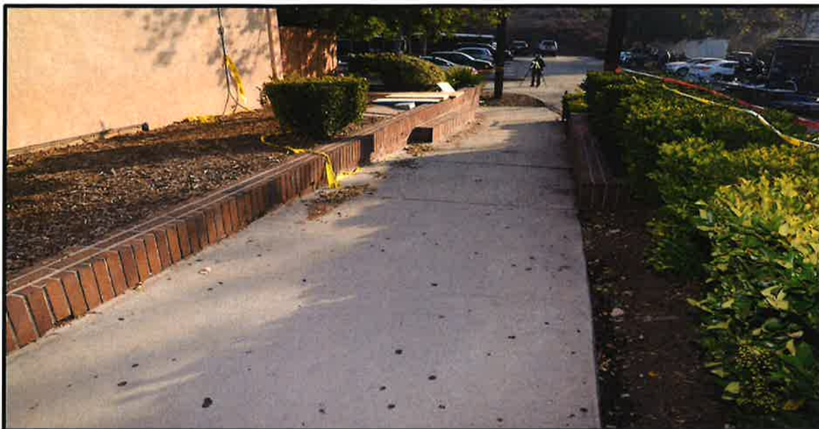
Concrete sidewalk/walkway that stretches east and west along the south side of Borderline. This photo depicts the area east of the front doors/main entrance.
